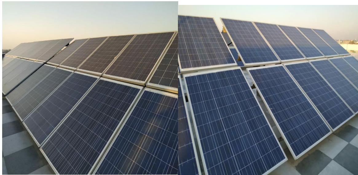
J1 – Solar Panels at IITM
