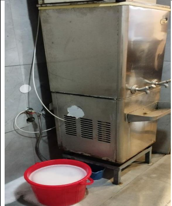
D2- RO residual collection for cleaning purpose
