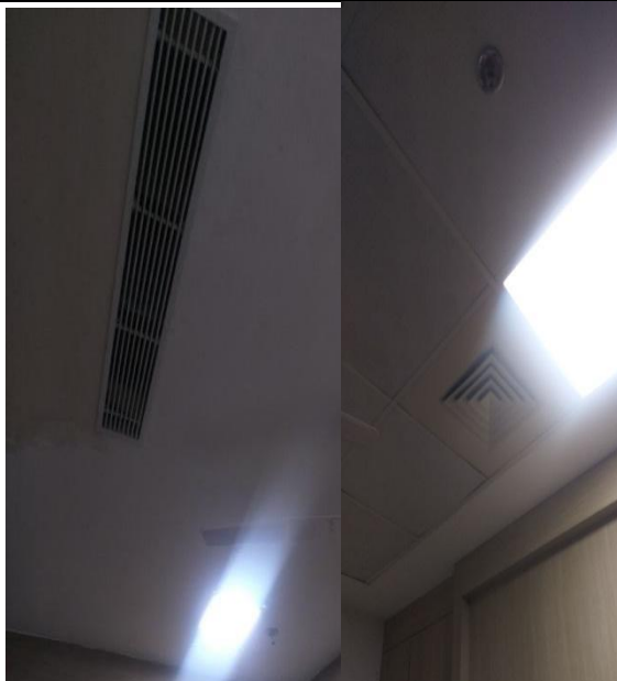
C3- Ventilation System
